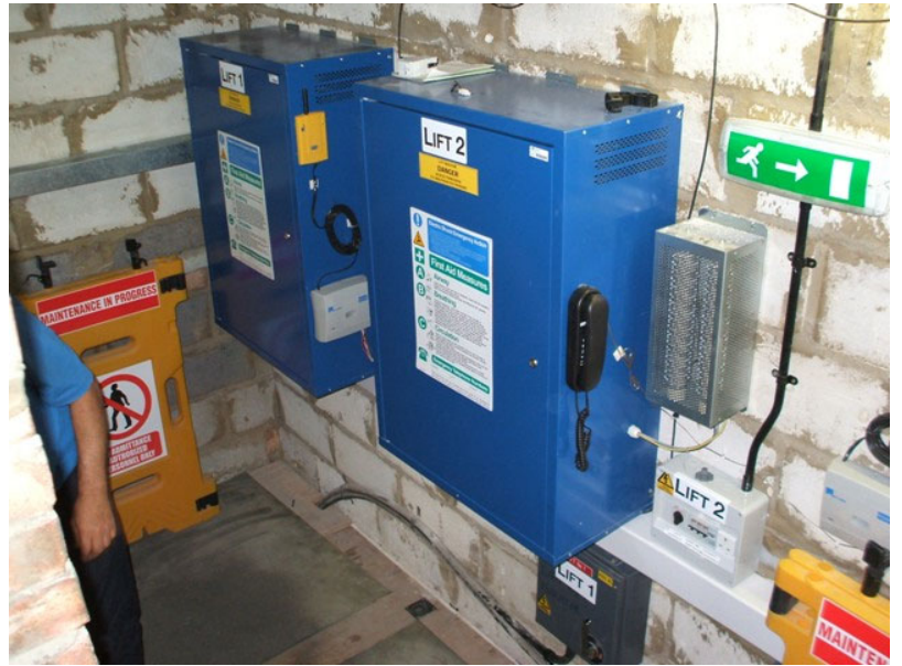
DUPLEX ARRANGEMENT UPTO 4 LIFTS CAN BE LINKED WITH SIMPLE CAN CONNECTION
